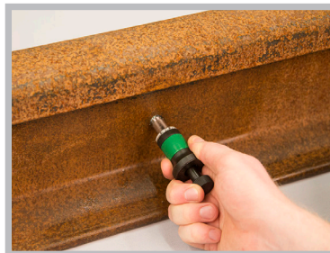
Screw Railbond on to the front of the assembly tool and insert it into the freshly drilled hole.
